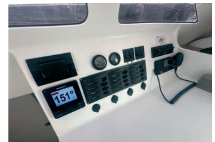
The helm station is complemented by a small area serving as a chart table, desk, and electrical panel.
